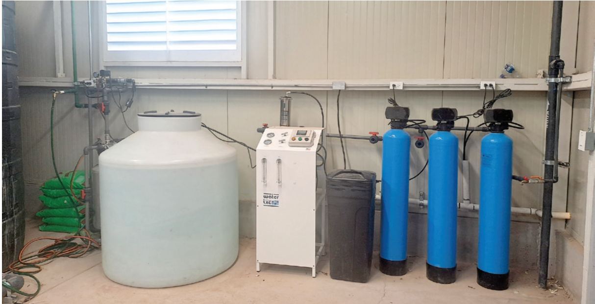
Water purification system in the Mexico factory
